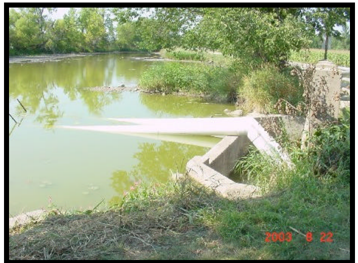
Siphons in place at the Geneva Lake water control structure, August, 2003.
